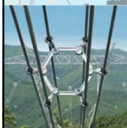
AEP 765 kV Interstate project
