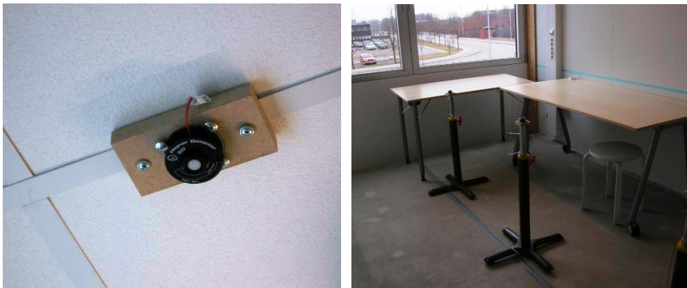
Figure 3.10 Ceiling mounted light sensor/sensors at table height (right).
