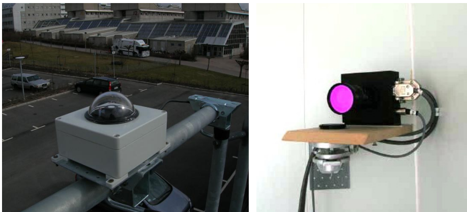
Figure 3.11 Outside sensor for global illuminance and luminance camera (right).
