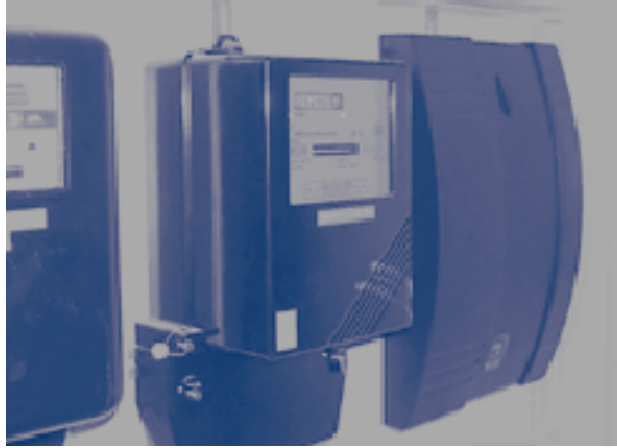
Figure 10.9: Oneline Box and an Electricity Meter [64]
